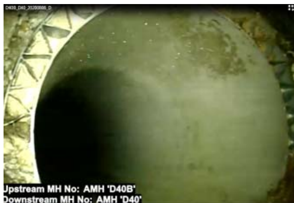
End view of PVC "truss" pipe. Can see the mortar deteriorating in the truss pockets.
