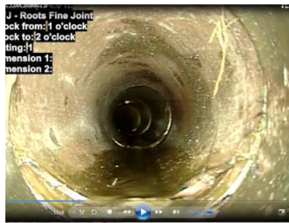
Broken joint in 6" VCP, starting to offset.
