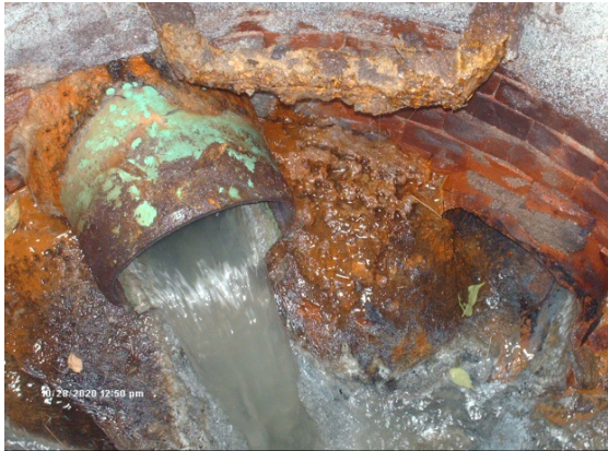
Infiltration through walls, mineral deposits.
