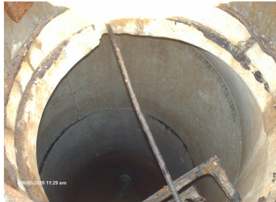
Utilities bore cables through manholes, breaking walls and chimney sections.
