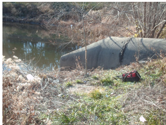
Manholes near ponds or ditches need to be raised to limit leakage from flooding.
