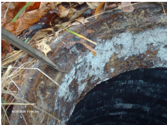
Cast iron frames rust and lose groove over years, making poor fit with lid.
