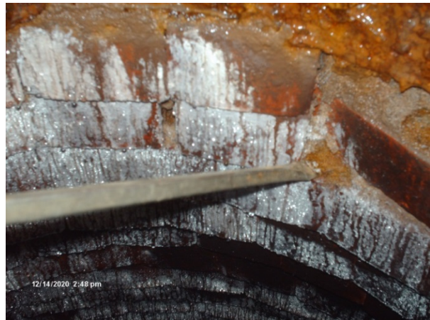
The bricks themselves become soft, from prolonged H2S-MIC corrosion.
