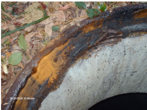
Severe corrosion on casting, losing structural shelf. (Nat. Sanctuary)
