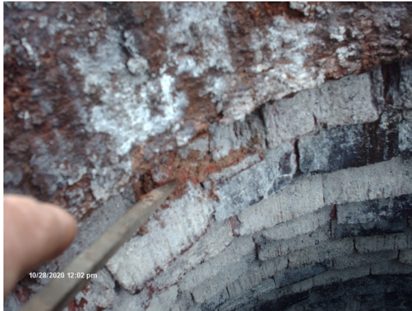
Mortar soft and crumbling, from H2S-MIC corrosion.
