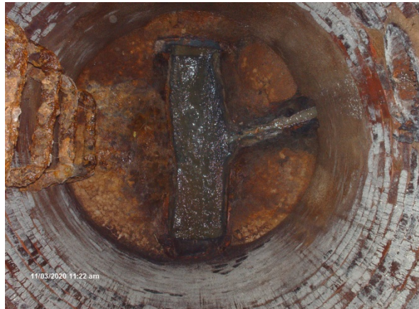
Some manholes have a concrete wall section below the brick, both corroded and soft.
