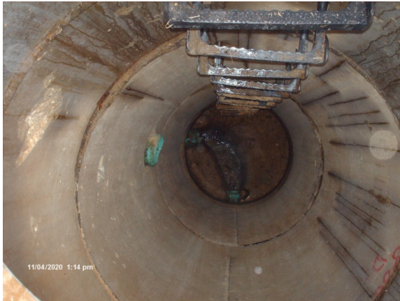
A "healthy" pre-cast concrete manhole. Note the gray color and smooth surface.
