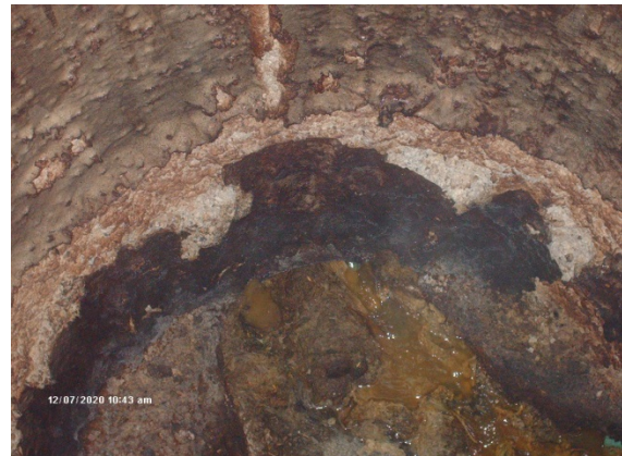
Advanced wall corrosion (H 2 S / MIC), by Price Chopper.
