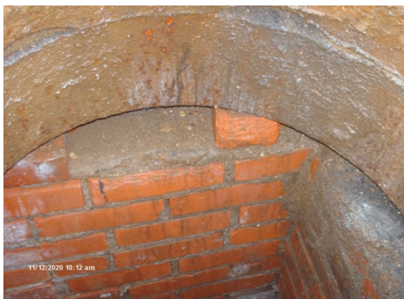
Typical brick "box" MH, in Hwy 9. Some bricks are falling away.
