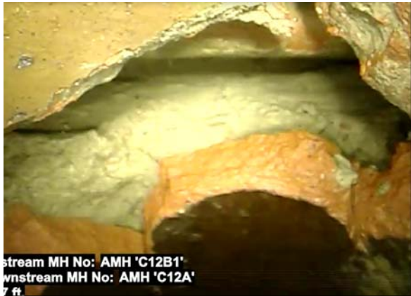
Bored cable broke away top of clay sewer pipe.
