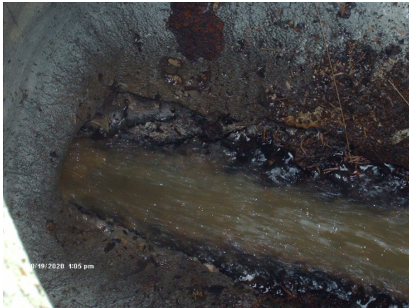
Corrosion undercutting bench, in previously lined manhole. (Wht. Aloe Nat. Sanctuary)
