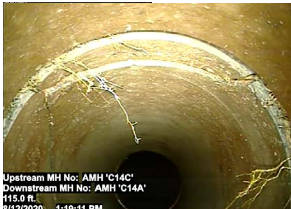
Broken joint with roots coming in, 6" VCP.
