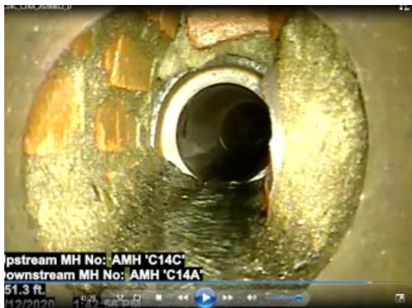
Old brick junction box, buried, in 6" VCP. This will need to be removed and replaced prior to CIPP lining.
