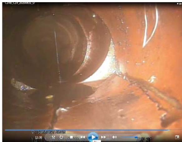
Broken 6" VCP under road, with infiltration runner.
