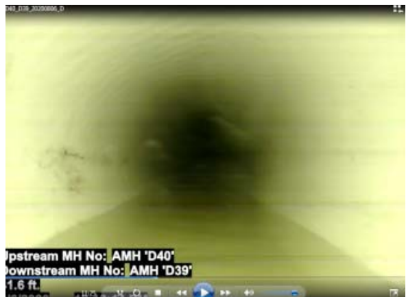
8" PVC pipe in good shape, but line has sag, will need jetter cleaning periodically. (Line was laid with no slope.)
