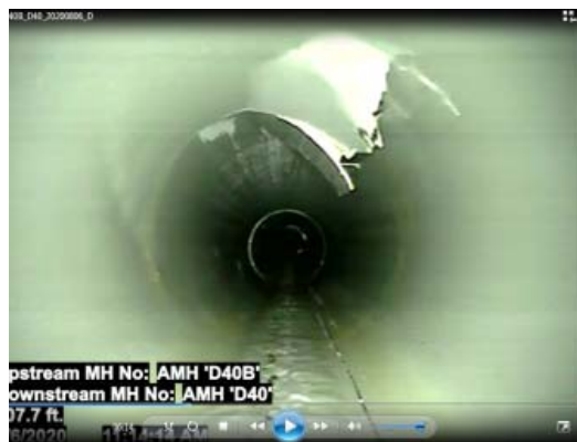
Hole in crown of PVC "truss" pipe. Can see the thin inner skin broken. Likely done during installation.
