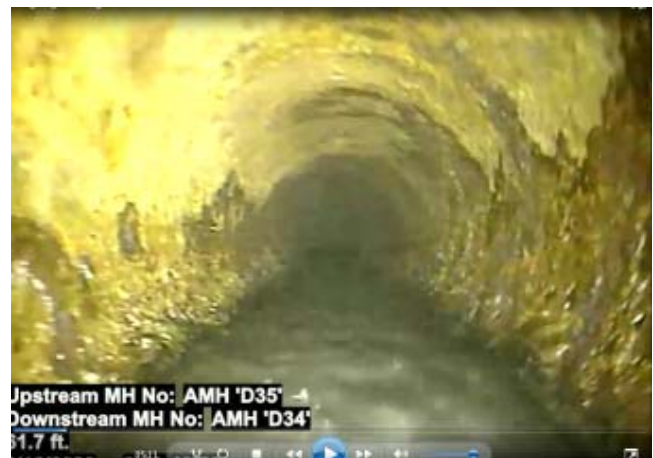
8" iron pipe (under Comm. Ctr. Lot) corroded and spalled.
