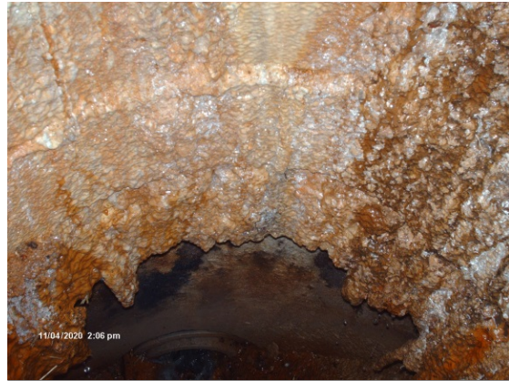
Infiltration through chimney, heavy mineral deposits.
