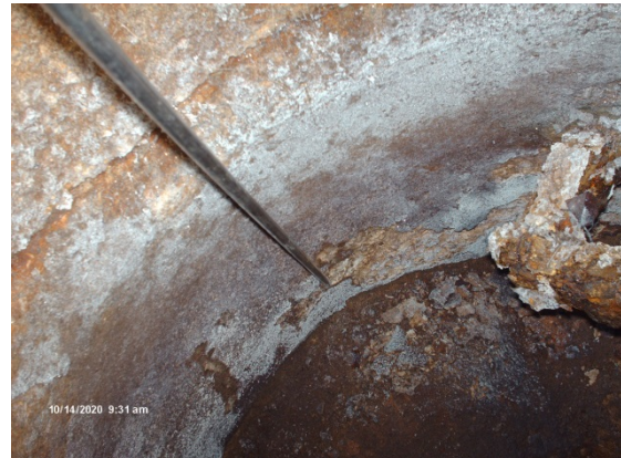
Moderate wall corrosion (H 2 S / MIC), the Bluffs.
