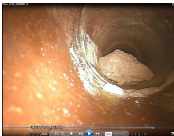
Rock inside 6" VCP, blocking camera.
