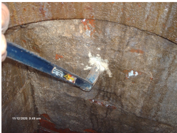
Mortar becomes soft, crumbles. (75 yrs old.)
