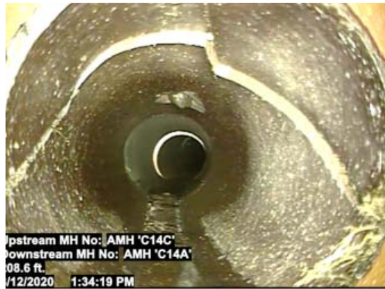
Spiral fracture, with offset movement, 6" VCP.
