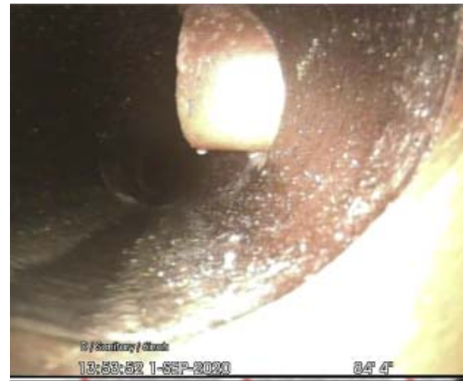
Intruding lateral pipe, need to trim.
