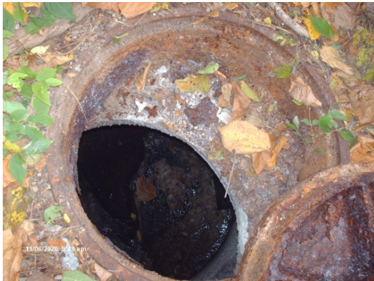
Lid offset on cone, moved by grading work or by shifting earth.
