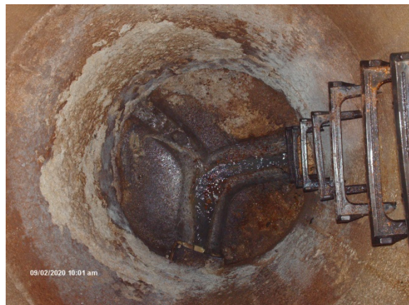
Heavy wall corrosion after 15-20 years – from forcemain discharge (River Hills).
