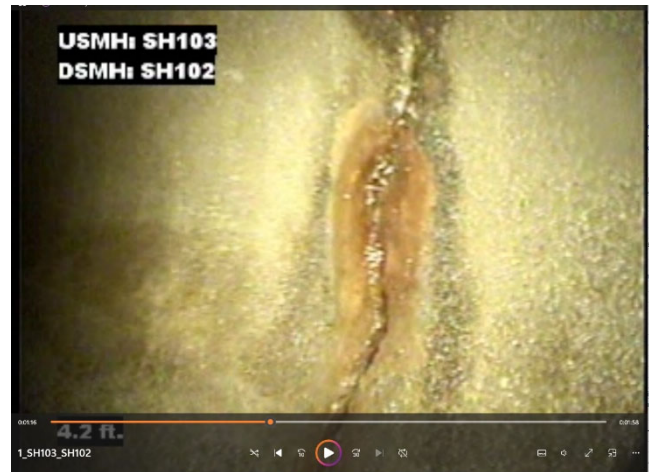
View of invert of RCP culvert SH103-SH102. Circumferential cracks in pipe wall, allowing reinforcement to corrode, soil to enter.
