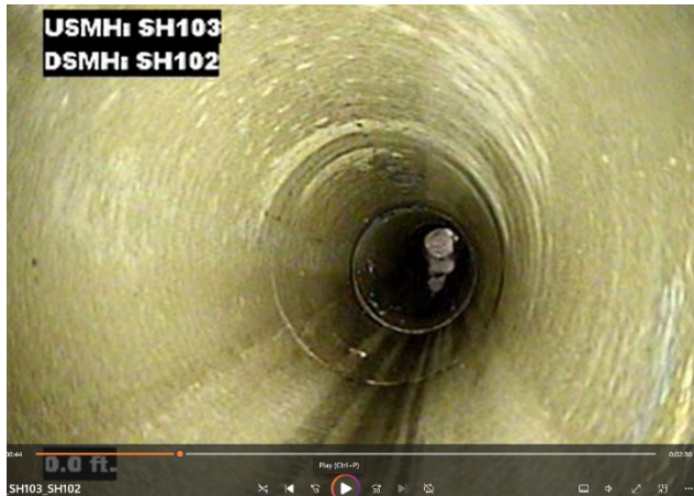
View of invert of RCP culvert SH103-SH102. Circumferential cracks in pipe wall.
