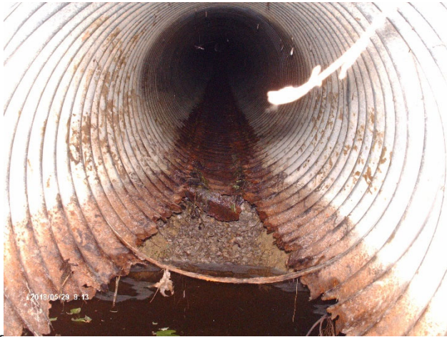
View invert of CMP culvert SR190-SR189. Culvert bottom is heavily corroded, has holes, allowing water to under-cut the bedding.
