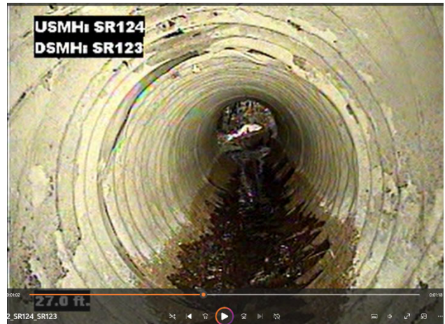
View invert of CMP culvert SR124-SR123. Culvert bottom is heavily corroded, large holes in bottom.
