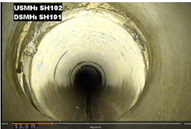
View of invert of RCP culvert SH102-SH101. Culvert large gaps at joints, broken concrete, soil washing into pipe.
