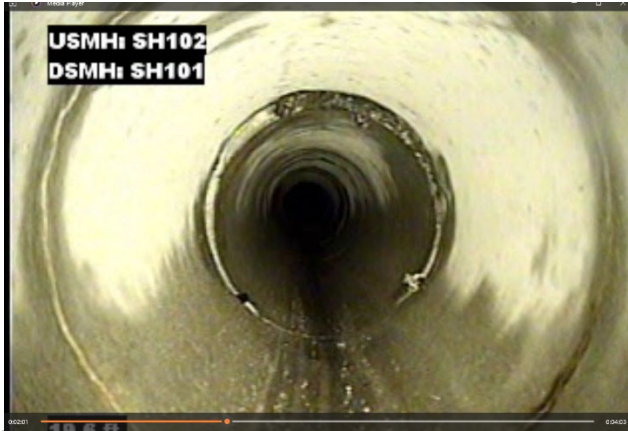
Same RCP culvert SH102-SH101. View of circumferential cracks in pipe.
