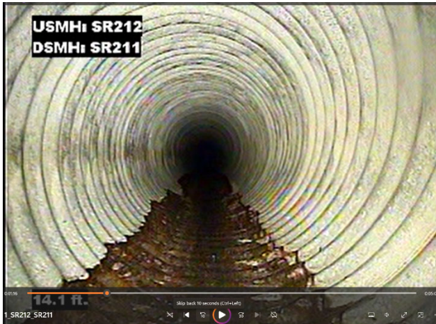
View invert of CMP culvert SR212-SR211. Culvert bottom is heavily corroded.
