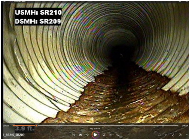
View invert of CMP culvert SR210-SR209. Culvert bottom is heavily corroded.
