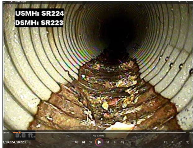
View invert of CMP culvert SR224-SR223. Culvert bottom is heavily corroded. Holes in bottom are catching debris.
