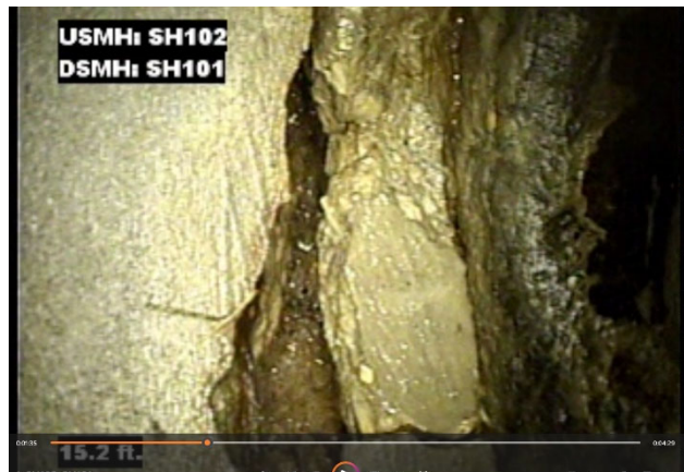
Same RCP culvert SH102-SH101. View of broken and open joint.
