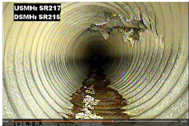
View invert of CMP culvert SR217-SR215. Culvert bottom is heavily corroded, pipe has gash in top, can be repaired using CIPP.
