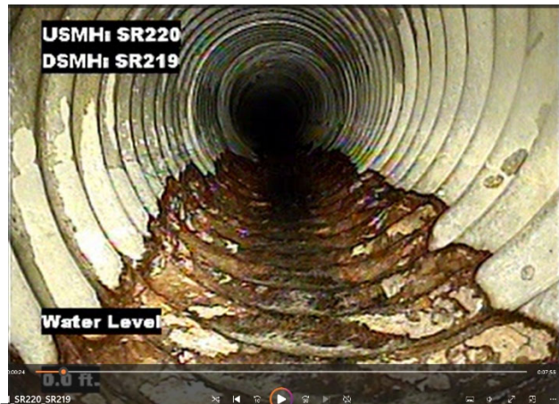
View invert of CMP culvert SR220-SR219. Culvert bottom is heavily corroded.
