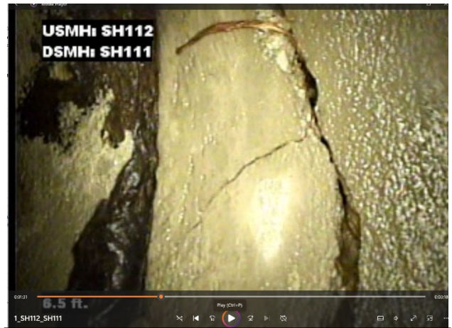
Same as left, RCP culvert SH112-SH111. Cracks where joint is broken.
