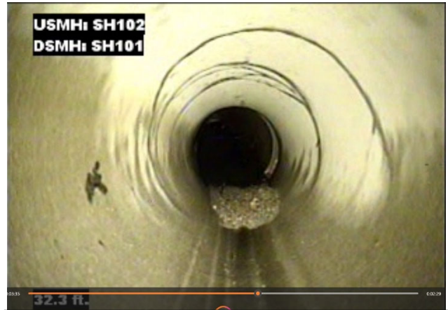
Same RCP culvert SH102-SH101. View of circumferential cracks in pipe, also open joint allowing soil to enter.
