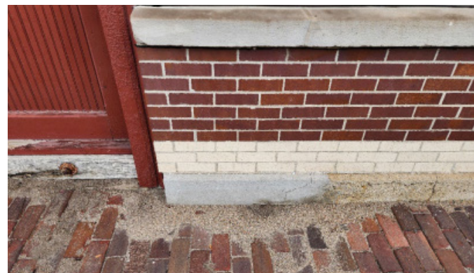
Water currently flows toward the structure due to inadequate site grading. The structure shows signs of past foundation repairs.
