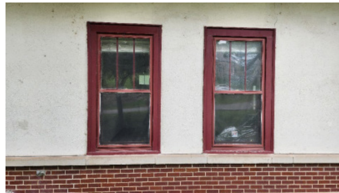
Multiple windows show sign of weathering and deterioration, as well as past repair efforts.
