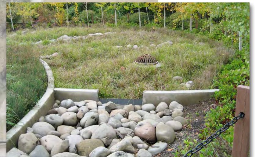
Green stormwater infrastructure
