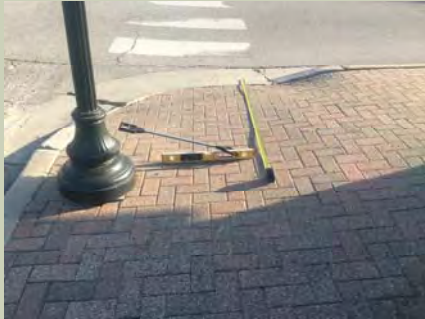
Truncated Domes Missing
