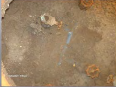
Mud and water wash into pit, accelerate corrosion.
