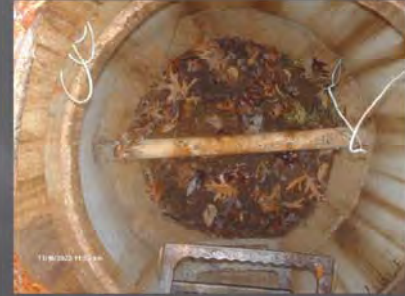
Valves never installed.... Can't isolate sections.
