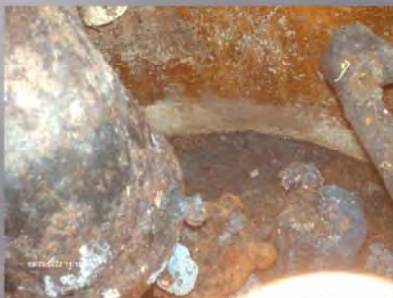
Gas corrosion of concrete.
