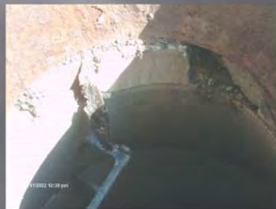
Broken chimney rings.
