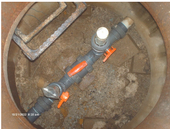
In-line clean-out pit, with mainline valve and riser valves, smaller diameter, newer PVC.
