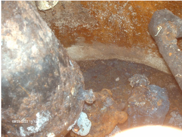
Corrosion to concrete, from gases released from air/vac valve. Needs to be lined.
