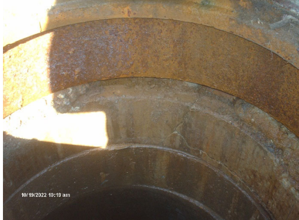
Holes in chimney, from concrete crews.
