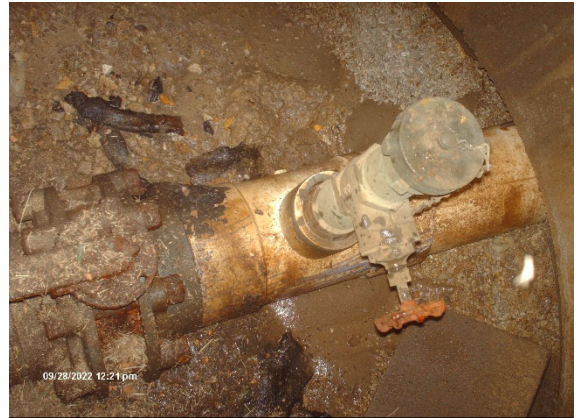
Leak in pipe fitting, sewage seeping out.
