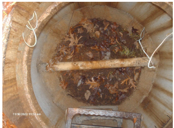
Valves are missing! Were never installed. West Shore Estates. Several like this....
