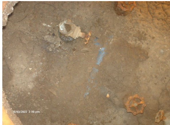
Mud fills bottom, accelerates corrosion and makes operation difficult.
