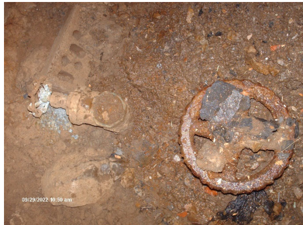
Valve bodies and handles rust away. These from early 1990's.
