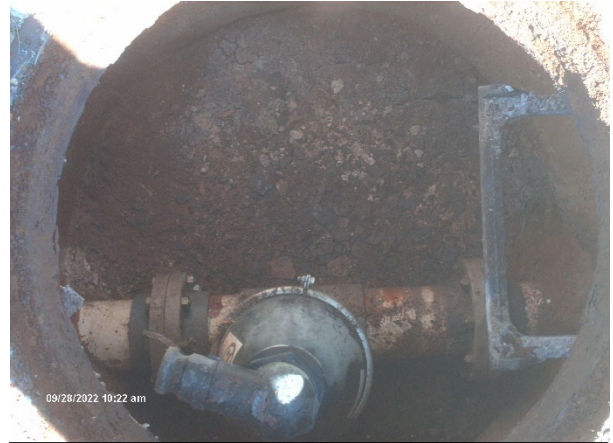
Air valve pit., with A.R.I. type air/vac valve and isolation valve below.
