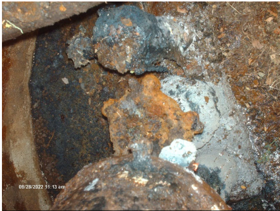
Valves seized up and coated with corrosion. Needs total replacement.
