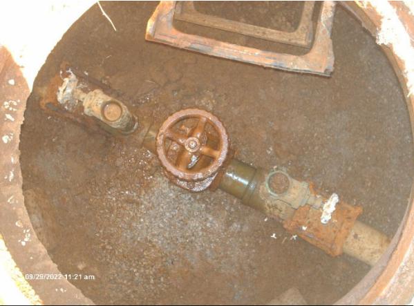
In-line clean-out pit, with mainline valve and riser valves, larger diameter, metal valves.
