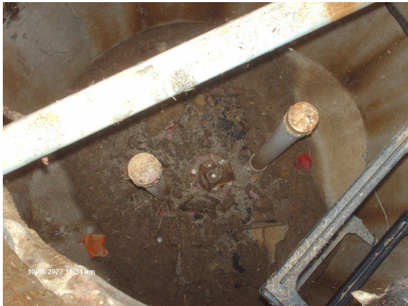
Utility pipe or conduit bored through pit. Needs to be relocated.
