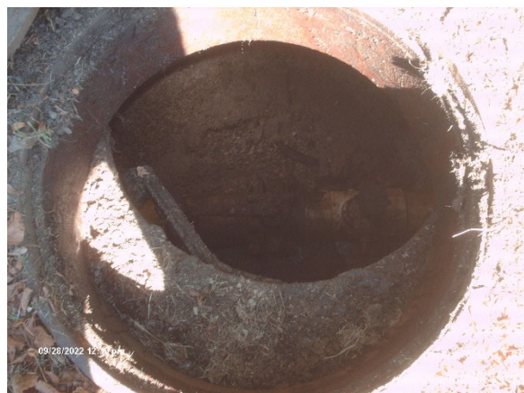
Casting shoved over on cone – makes access impossible.
