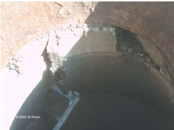
Broken chimney, admits mud and gravel.
