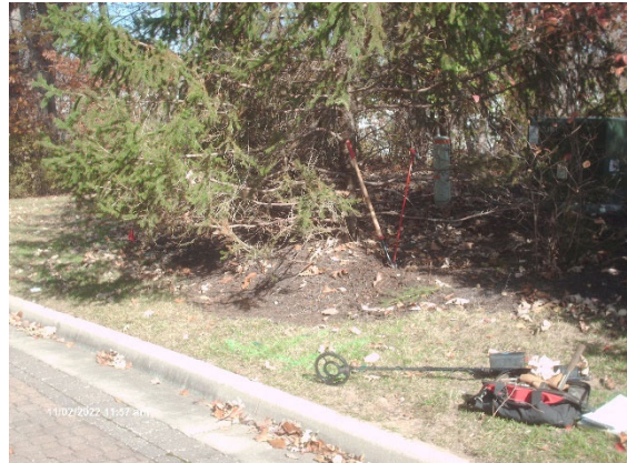
Pine tree planted on top of valve pit lid, will require tree removal.
