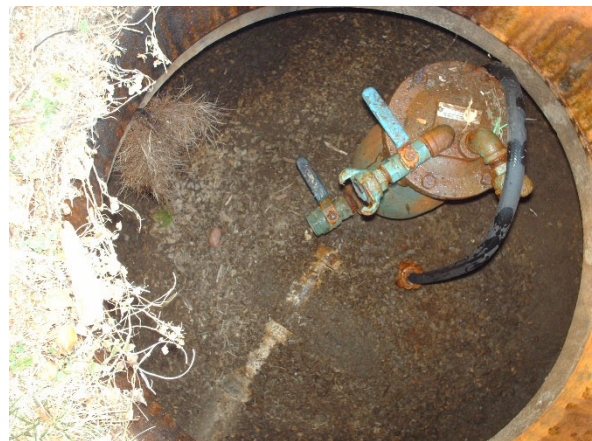
Air valve pit, with old cast-iron air/vac valve. These corrode badly.
