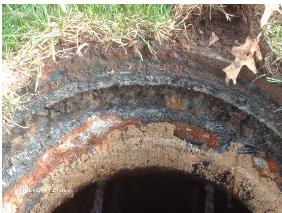
Severe corrosion on casting, from gases. Lid welds to frame. Needs non-metallic.
