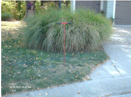
Clean-out pit buried below turf. Usually 6 to 8 inches deep.
