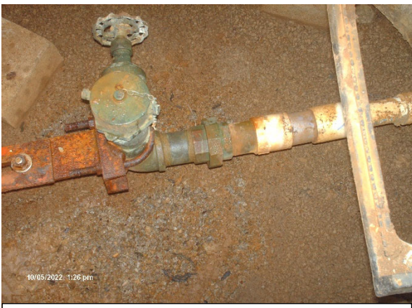
Older end-of-line clean-out pit, with brass valve and steel strut.
