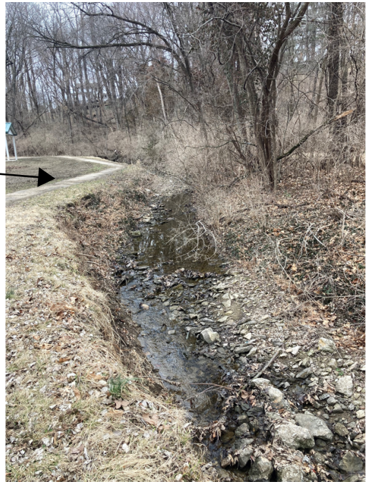
CREEK BANK LOOKING WEST (stabilization required on left side)
