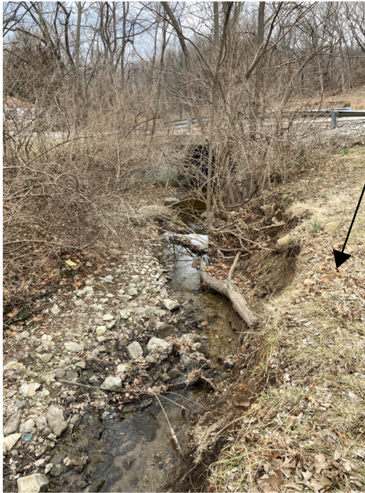
CREEK BANK LOOKING EAST (stabilization required on right side)
